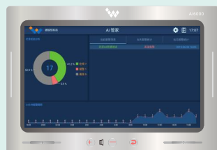
Central Alarm Controller
